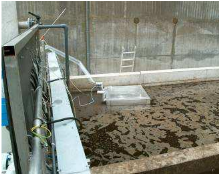
Picture 2. Lindvall box at the surface of a denitrification tank
